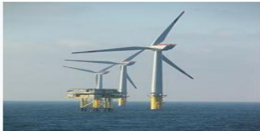
Fig: 4. Wind turbines and electrical substation of Alpha Ventus in the North Sea
