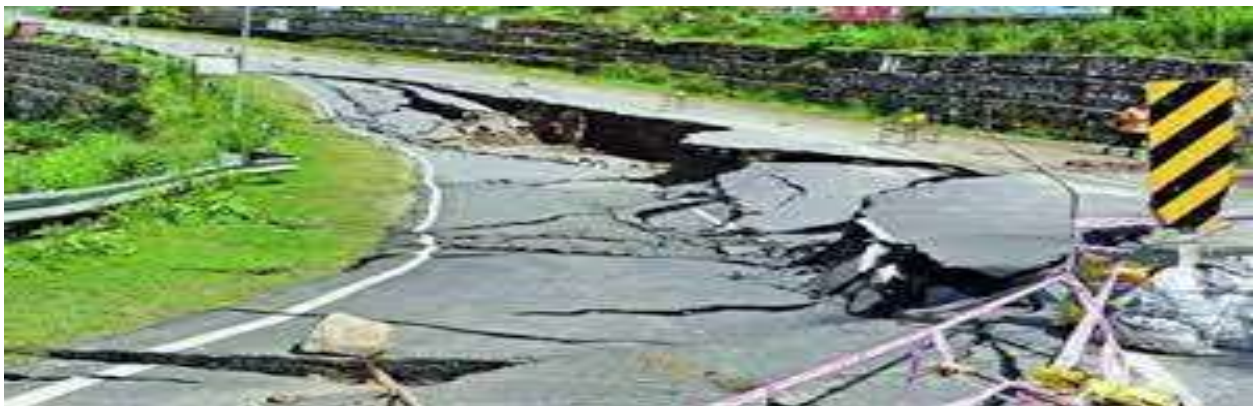
Fig. 3 - Stretch of Badrinath highway caves in, sinks by 3ft in 24hrs
