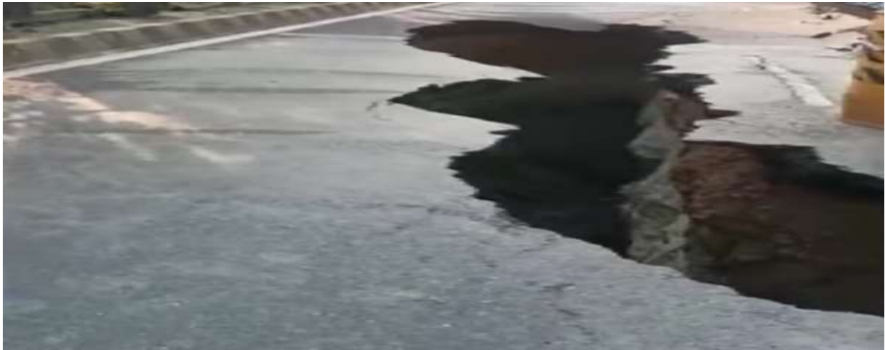
Fig. 6 - Noida-Greater Noida Expressway collapse
