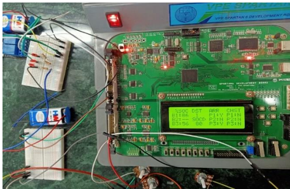
Fig.8 Complete of charging process for EV1
