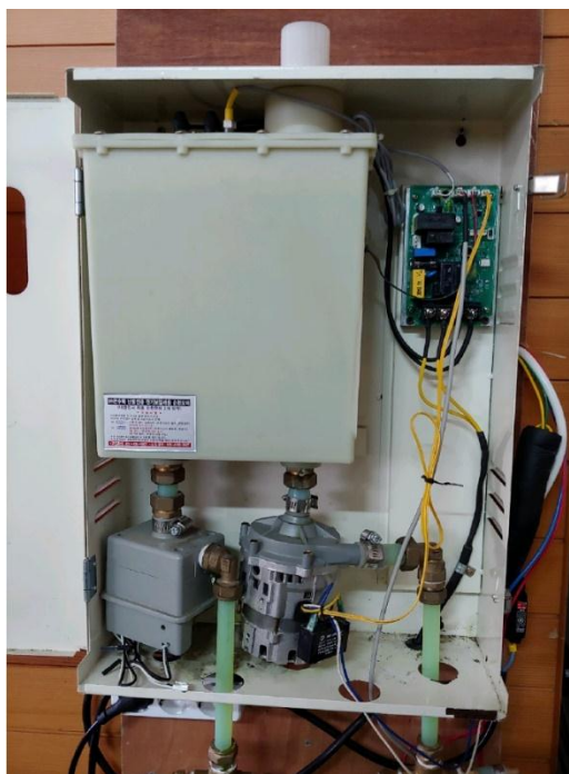
Fig. 3 A hot water boiler to supply thermal energy to a small two-person pension
