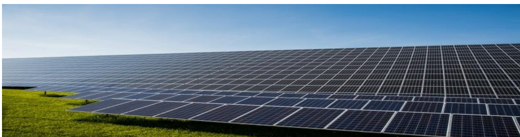
Fig.3 - Solar energy the eco-friendly form of energy.
